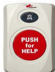
R4KPB12 Push for Help Station
